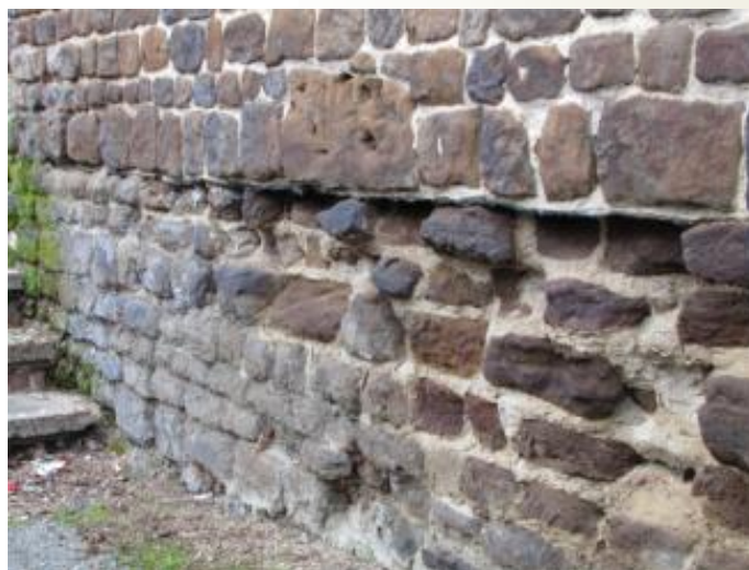
Eroded stonework on the south wall of the Hall.
